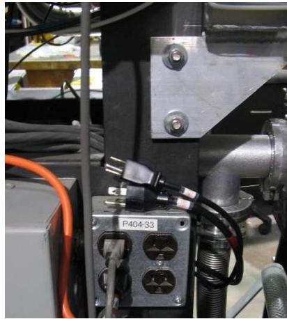
Figure 4.11: Turn off the switch box of the South and the North bender
